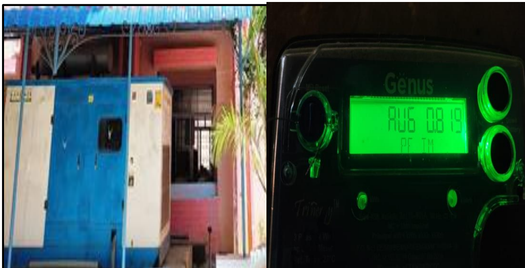
Energy conservation facilities observed in the Campus
