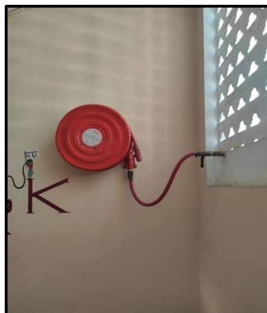
Fire Safety measures designed at the Campus to ensure the Safety of the Stakeholders
